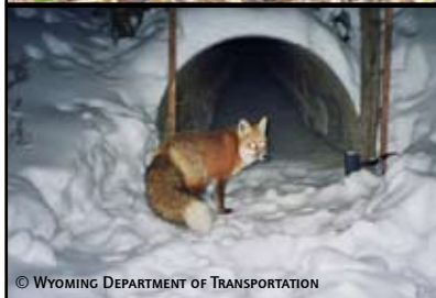
PINE MARTEN (TOP) AND RED FOX (BOTTOM) USING A ROUND CULVERT ON US 287/26 EAST OF TETON NP IN WYOMING ON THE TOGWOTEE PASS HIGHWAY.
